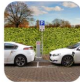
EV Charging Spots
